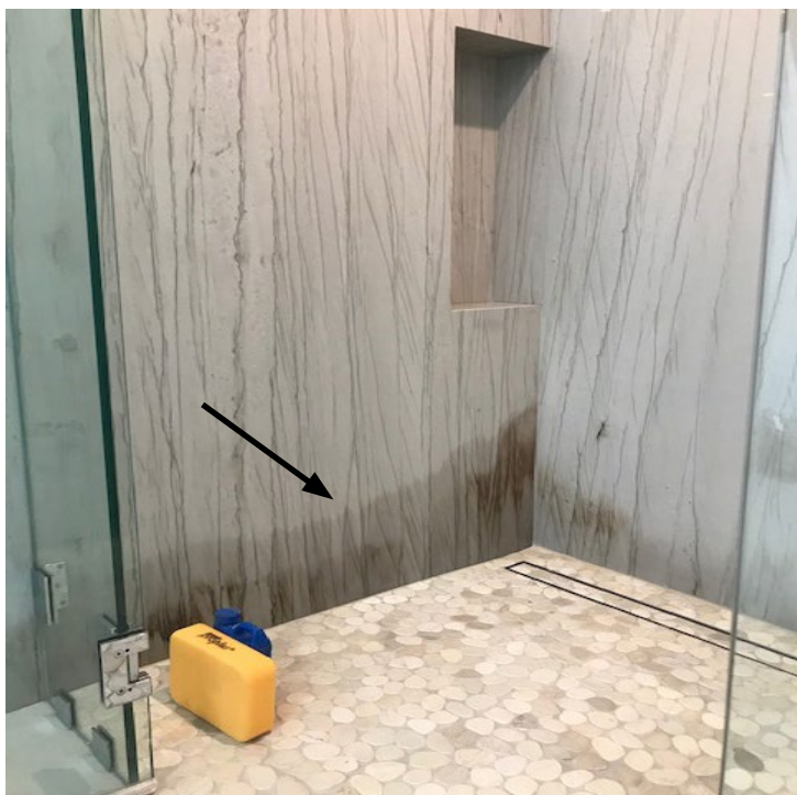
Water intrusion in a shower. Sealing front and back of natural stone is very important.
